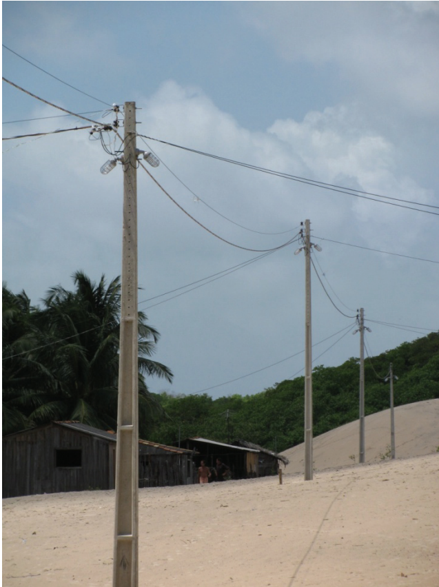
Fig. 7 View of the aerial distribution network.
