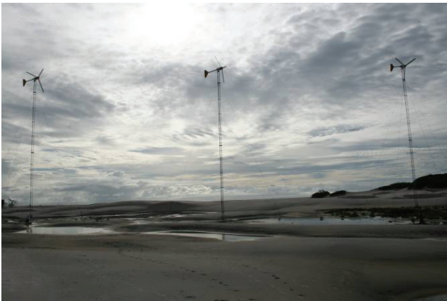
Fig. 5 Wind turbines installed in the island
